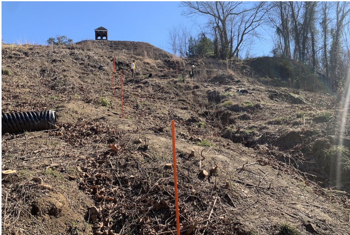
Karen and Quincy, and Lynne and Piper working on the steep landslide portion of the work area.
